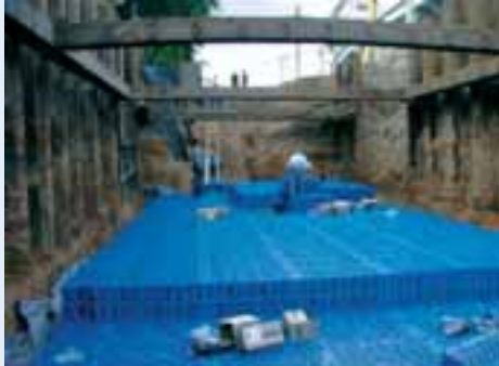
Infiltration system at Frankfurt stadium.
