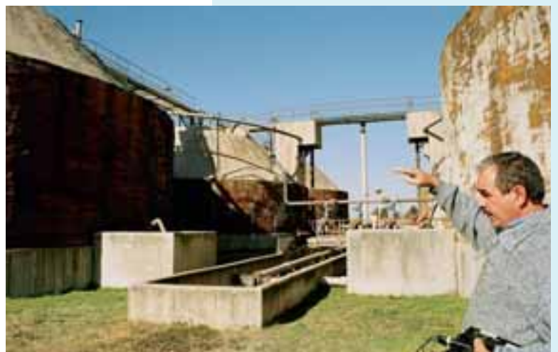
Sewage plant near Sebokeng Township close to Johannesburg, South Africa
