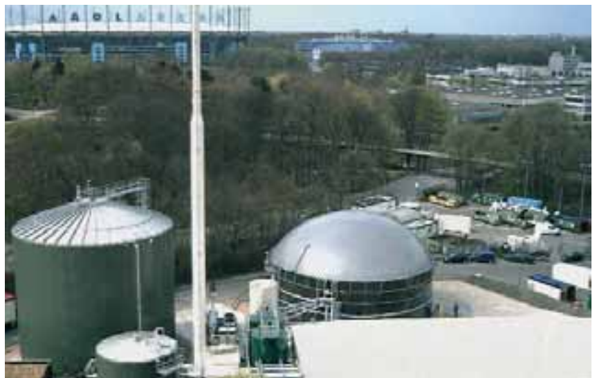
Hamburg stadium covers its demand for heat from a nearby biogas plant.
