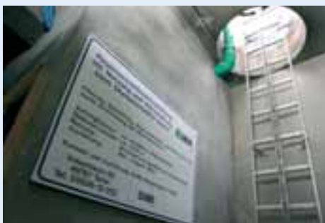
Interior view of the rainwater cistern at the Olympia Stadium in Berlin.
