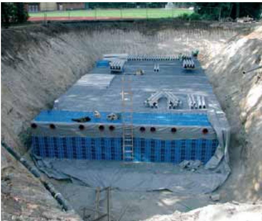
Underground infiltration plants - like here in Frankfurt stadium - store rainwater and let it slowly seep into the natural water cycle.
