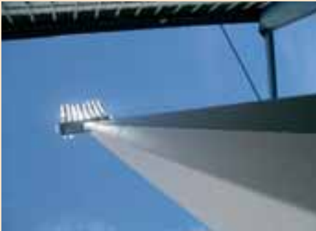
Floodlighting systems are the largest consumer of electricity in stadiums. Modern floodlights provide better illumination but use less electricity.
